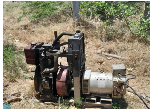
b) Well Motor: 3HP (1 Nos.)
